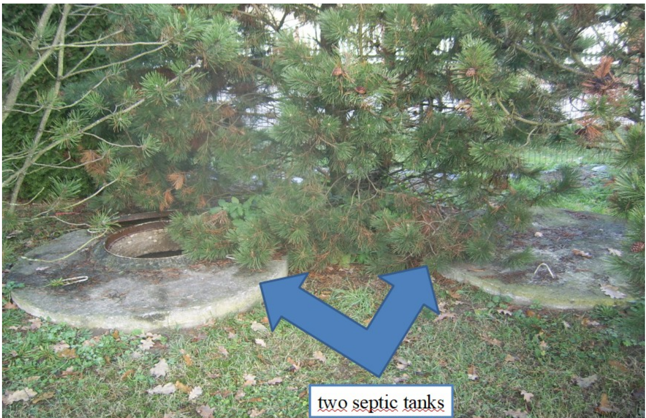
Figure 10. Two septic tanks next to the school in the village of Bruszewo in Sokoły municipality [own picture 11.2016]
