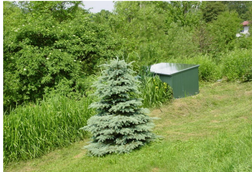
Installation with biological bed with rainy distribution of wastewater and with a special bed on a slope filled with soil and hydrophilic plants on an agrotouristic farm, according to ITP ZSIT GCB Tylicz project.
