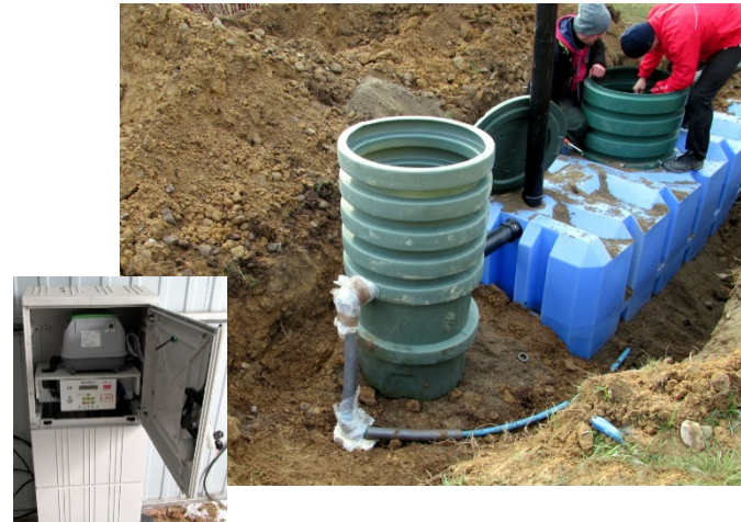
Example of household prefabricated hybrid SBHR treatment plant with activated sludge and with elements of biological bed immersed in wastewater. During installation.
