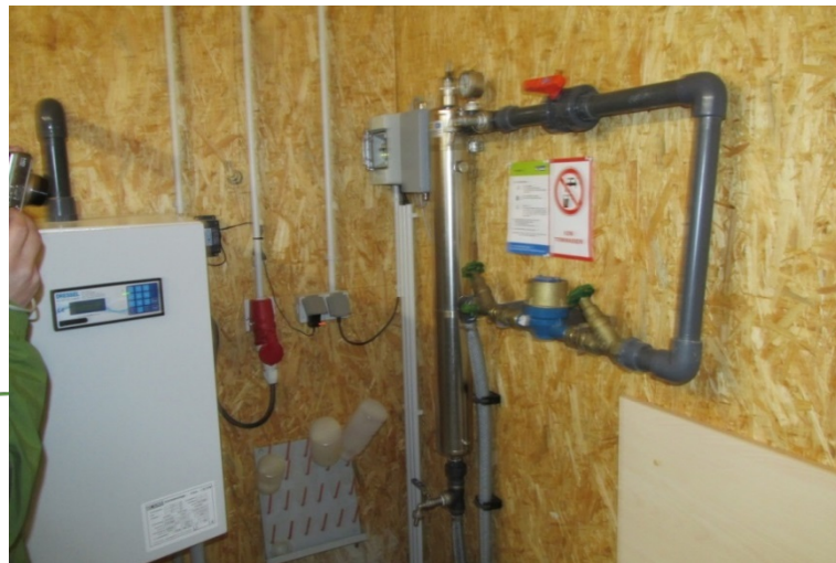
Example of installation for final disinfection of wastewater in local treatment plant (SBR type) using UV radiation
