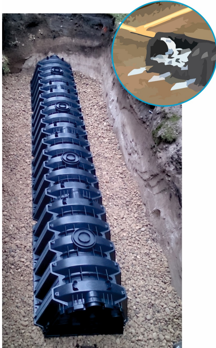
Figure 12. Infiltration fields consisting of infiltration tunnels under construction. Photo: A. Percovs. Figure: L. Urtāne
